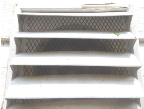
HRV intake requires cleaning
