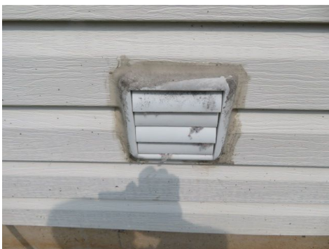
Dryer exhaust needs cleaning
