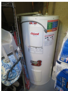
Giant electric hot water tank (40 gal)
