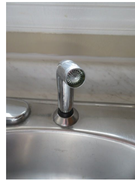
Kitchen spray wand not connected
