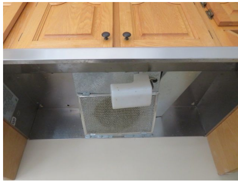
Range exhaust hood
