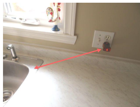
Non-GFCI receptacle within 1.5 m of kitchen sink
