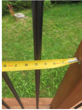
Deck baluster spacing exceeds max.4" in some places
