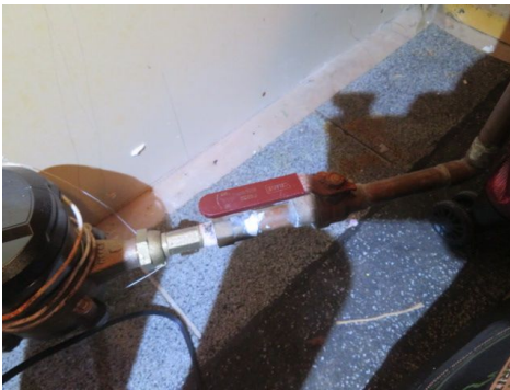
Main water shut off valve
