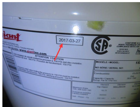
Hot water tank nameplate (2017)
