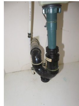
Main bathroom sink waste plumbing
