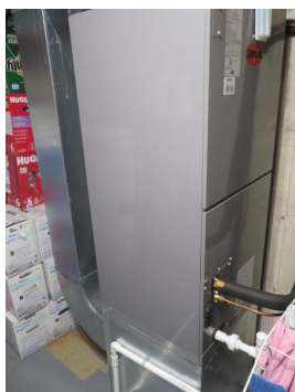
Forced air furnace
