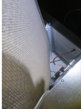
HRV exhaust filter dirty
