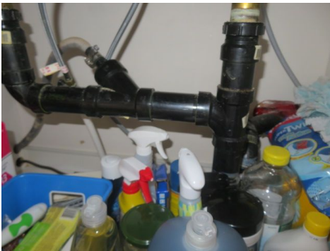
Kitchen sink waste plumbing
