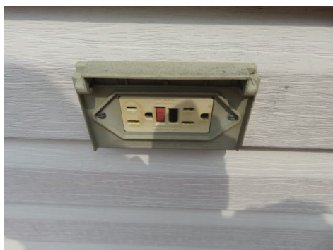
Rear exterior receptacle missing cover
