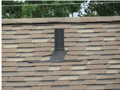
Plumbing vent stack
