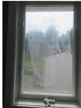
Main bathroom window seal has failed
