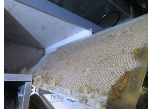
HRV intake filter dirty
