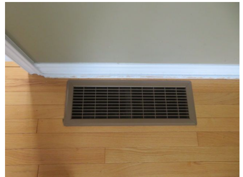
Main hallway return register
