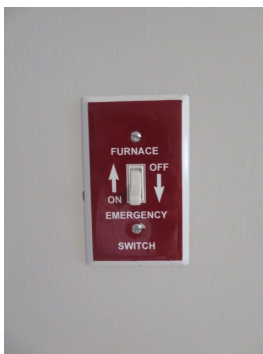
Furnace safety switch not required
