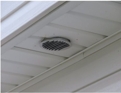
Basement bathroom exhaust
