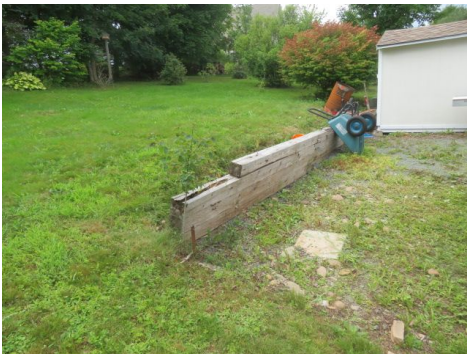
Rear timber retaining wall deteriorated
