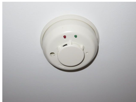
Heat detector on main floor
