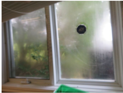
Garage window seal has failed
