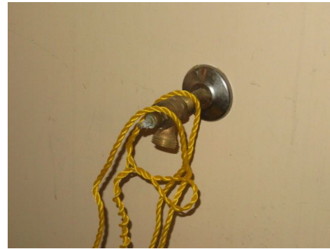
Hose bib in garage missing handle
