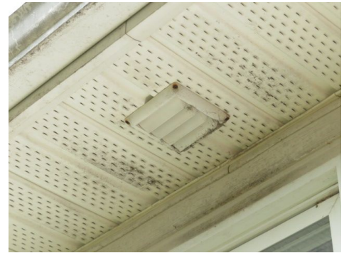
Main bathroom exhaust
