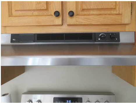
Range exhaust hood
