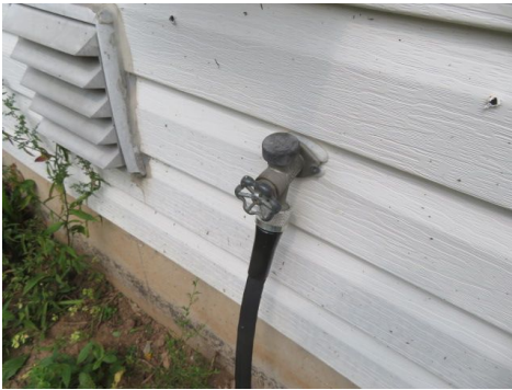
Frost free hose bib at rear
