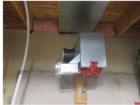
Induced draft fan for former oil fired furnace
