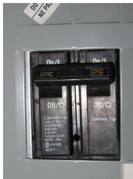
125 amp main disconnect
