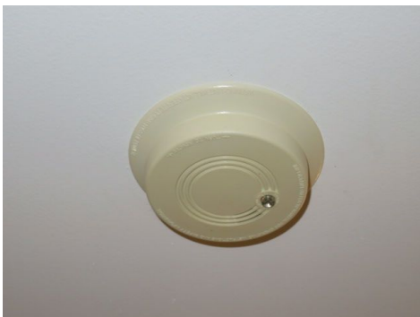
Basement detector outdated
