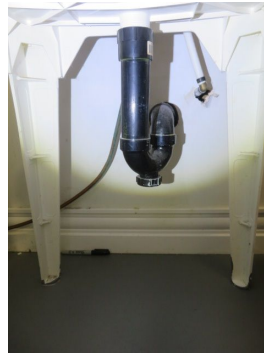
Laundry sink waste plumbing
